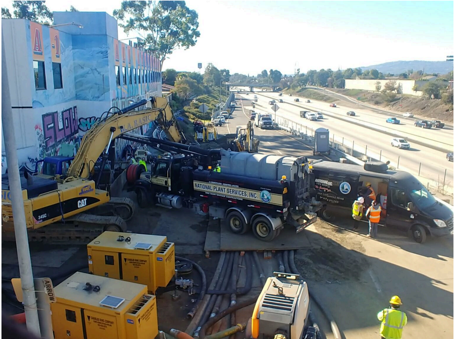
Crews work to address the site of a sewage spill, which discharged millions of gallons into the Dominguez Channel, at 212th Street in Carson on Jan. 2, 2022. Raw sewage first began overflowing on Dec. 30, 2021. Photo courtesy of the LA County Sanitation Districts.
