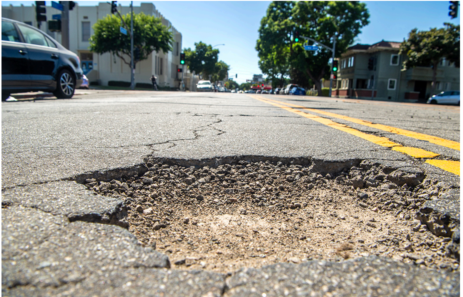
A pothole on Sixth Street near Lime Avenue in Long Beach, Thursday, Aug. 15, 2024. Photo by Thomas R. Cordova.
